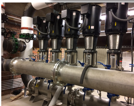
Left, five variable speed pumps circulate water from the 225 wells in the wellfield to the heating and cooling system in the Capitol.
