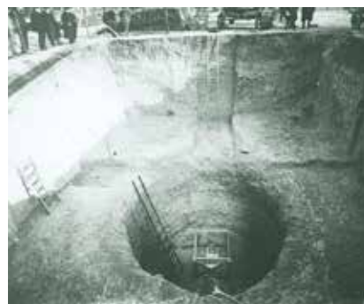
A square pit was dug to allow room for rails to be added. In the bottom of the pit a circular hole was dug to reach the Dakota Sandstone bedrock.
