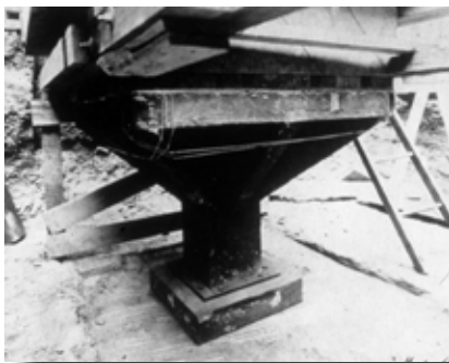
The punch rests on the sandstone at the start of the load test. The punch was used to focus weight and simulate the load of the building on the footings.
