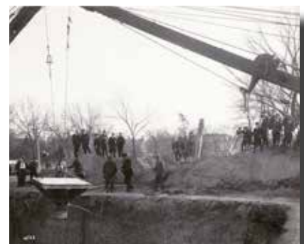
Once the sandstone bedrock was exposed, the punch was lowered into the hole and placed within the cribbing to await the addition of the rails.
